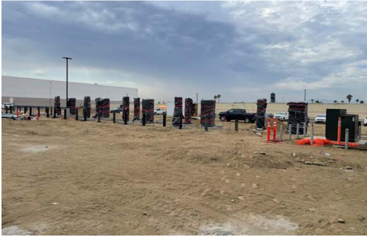
Installed chargers at Fleet A waiting to be energized, shared with permission from fleet
