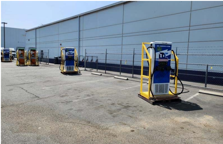
Skid mounted temporary 50kW chargers at Fleet C, shared with permission from DTNA
