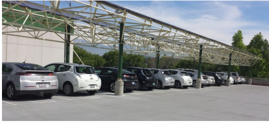
Figure 3. Level 2 EV Chargers Under the Solar Carport in the Upper Parking Lot Near the Employee Entrance
