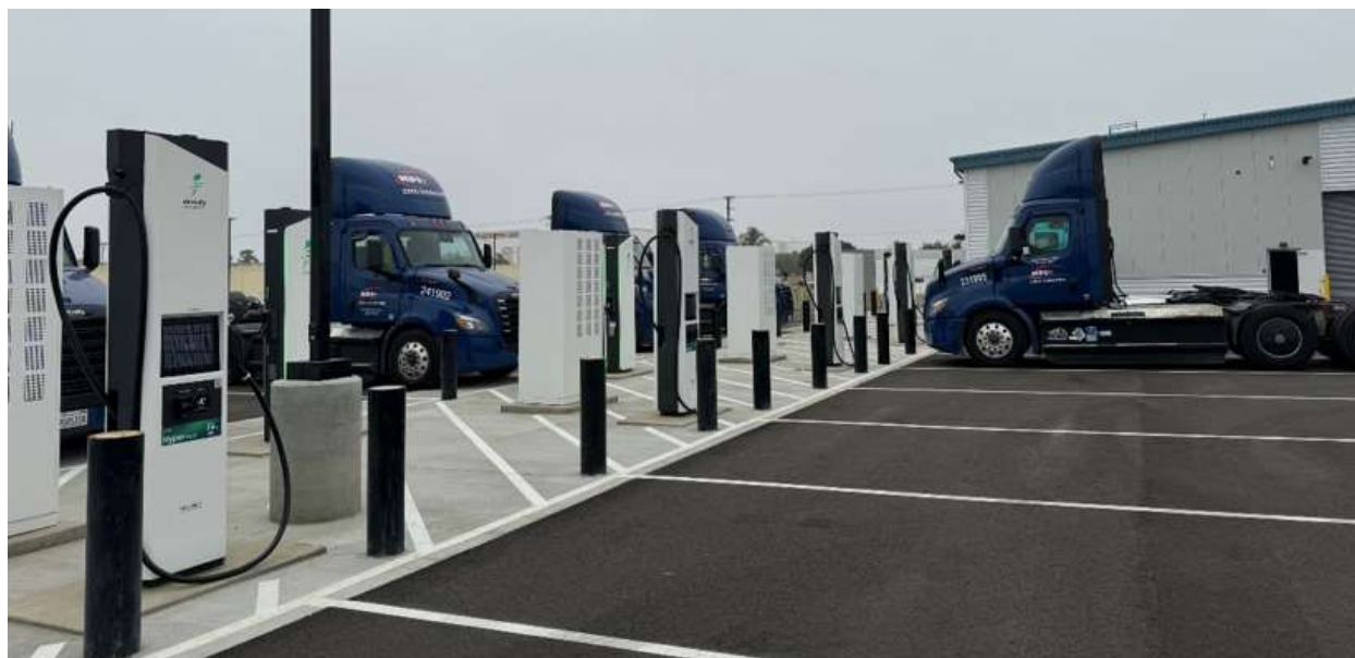
Figure 9: Partial Deployment of NFI Daimler Class 8 BETs and Charging Infrastructure
