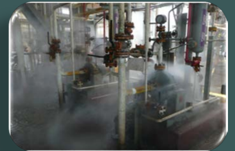
Water Spray for Pump Deluge
