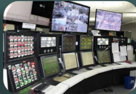
Control Panel for Water, Isolation Valves, and Acid Evacuation System
