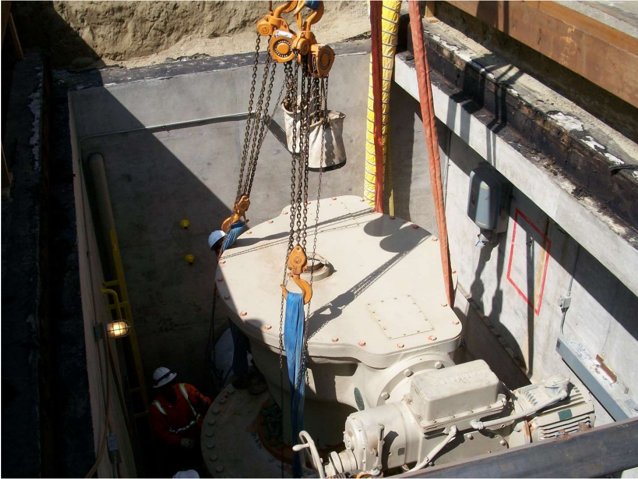
2. Inside view of the trench and vault (regular access would be via manhole)
