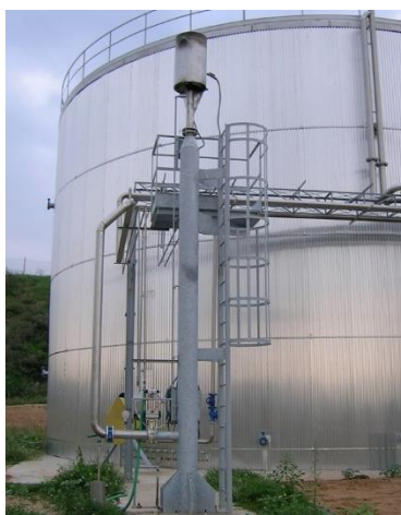
Figure 3-1. Non-Hydrogen Clean Service Flare (LPG Flare)
