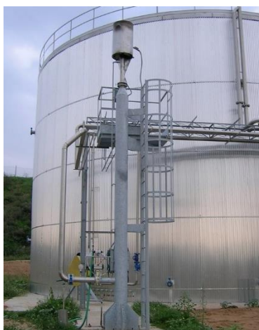
Figure 3-1. Non-Hydrogen Clean Service Flare (LPG Flare)
