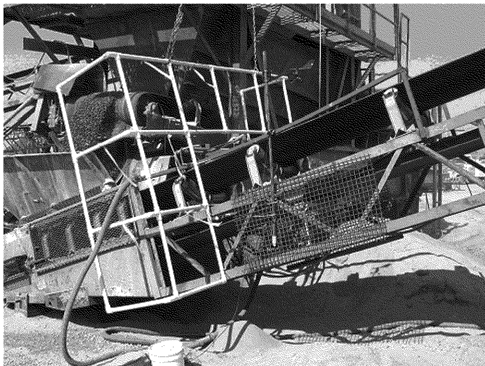
Figure 3. Close-up view of the sampling orifices in the conveyor transfer point array at the Carroll Canyon plant.
