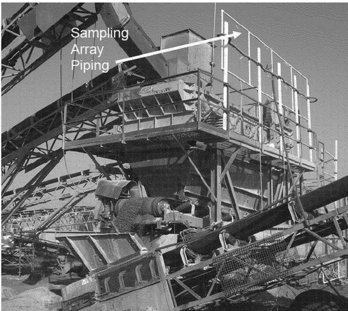
Figure 1. Side view of the sampling array on the downwind side of the vibrating sizing screen at the Barstow plant.
