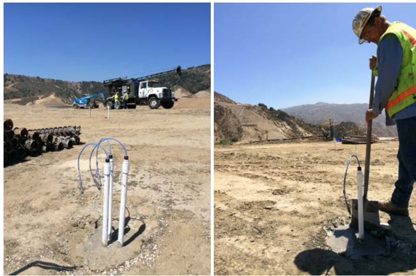
Photo 1- Shallow and deep vapor monitoring wells with pressure transducers installed.
