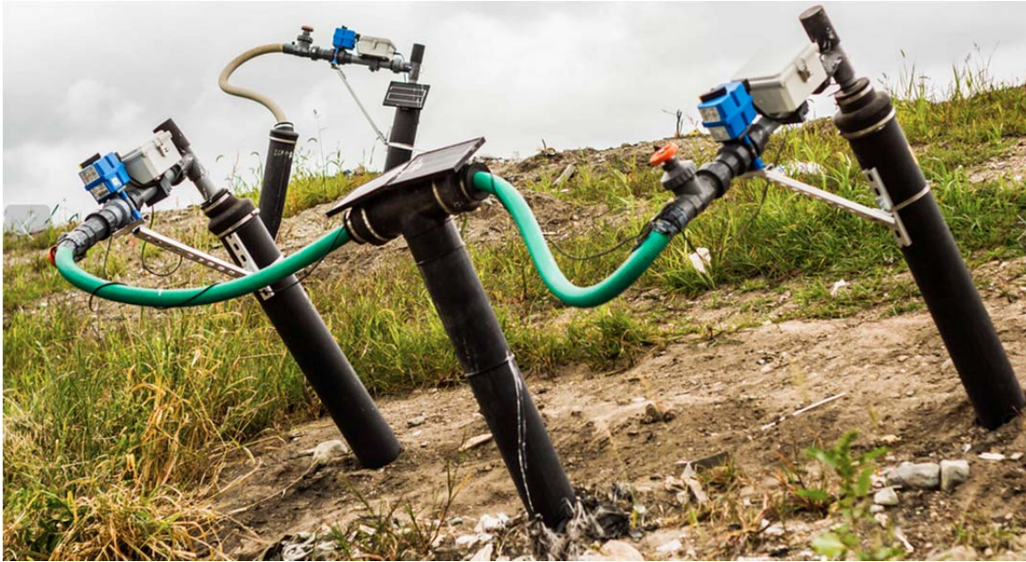
Photo 3- Loci Controls WellWatcher monitoring & control system used to automatically adjust and monitor each landfill gas well.
