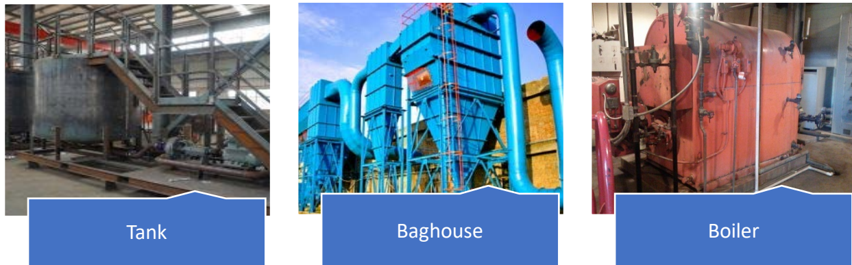
Figure 4-7: Examples of General Industrial Facility Equipment
