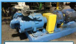
Stage 1 CM Pumps, Compressors
