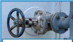
Stage 3 CM Valves, Fittings, Others
