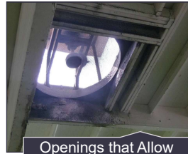
Openings that Allow Fugitive Emissions to Escape
