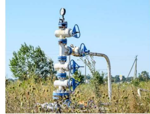
Example of an Injection Well
