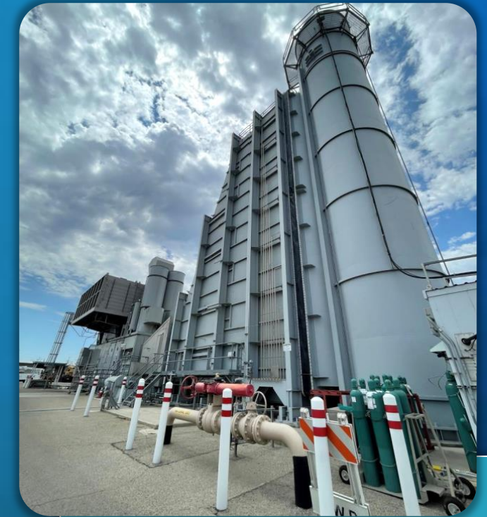
Industrial Combustion Boilers/Process Heaters/ Refineries/EGUs/Etc.
