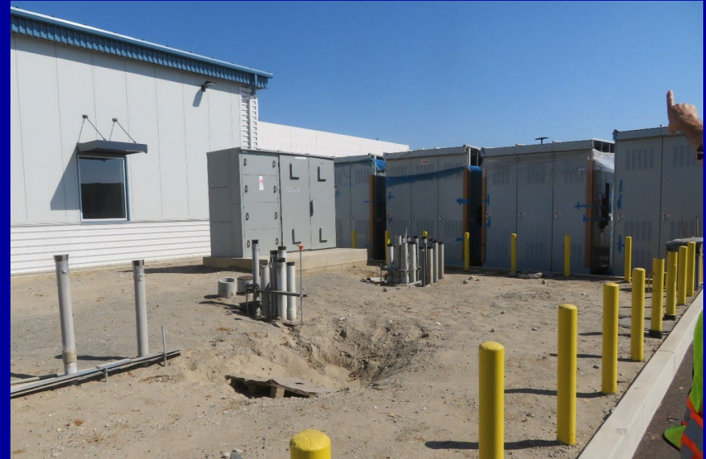
Infrastructure equipment to be installed at NFI fleet depot
