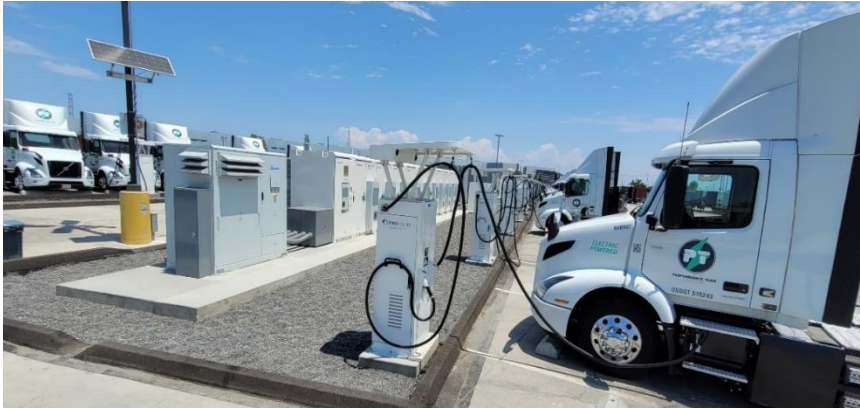
Figure 15: Class-8 EV truck charging at Denker Yard
