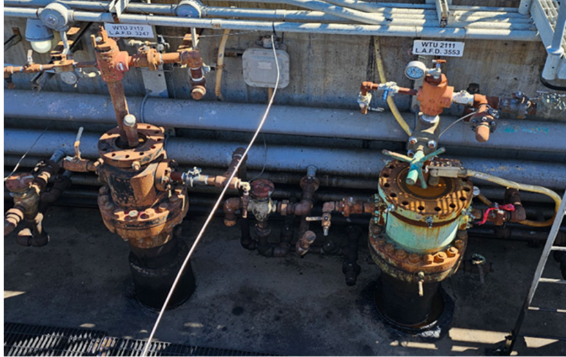
Figure 1.2 – Example of Wellheads Inside a Well Cellar
