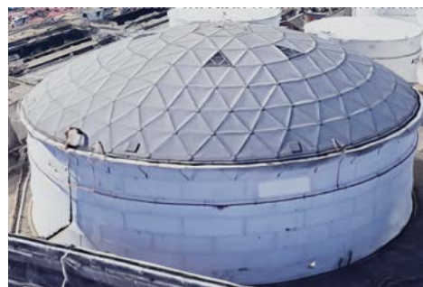
Figure 2-1- Domed Storage Tanks
